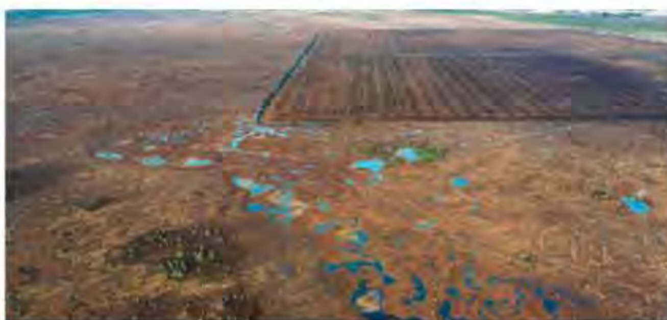
■ Figure D4.2.22 Drainage network establishment for peat extraction field, next to the natural peat bog wetland
